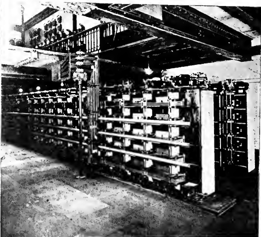
FIG. 15.—BUS-BARS, THIRD STATION.
